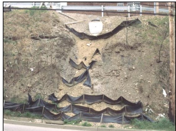
Figure 1 – Example of a Poor Installation
